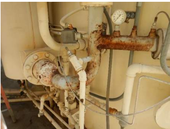
Photo 4-17. VANDA Level 2 condition on the lower piping leading to the Thaw Heater.
