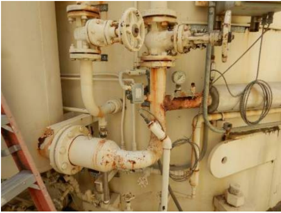
Photo 4-9. Typical VANDA Level 2 condition on the piping due to coating failures.
