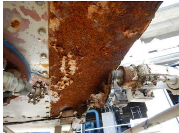
Photo 4-16. Detail view of VANDA Level 2 condition on the underside of the Turbine Duct.
