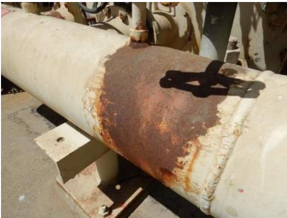
Photo 4-7. VANDA Level 2 corrosion on a manifold on the south side of the tank.
