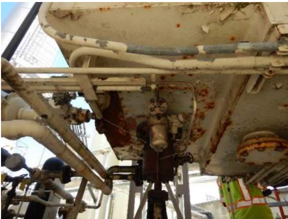
Photo 4-15. VANDA Level 2 condition on the underside of the Turbine Duct.
