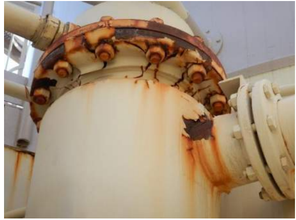
Photo 4-10. Typical VANDA Level 2 condition on the edges of the flanges, nuts, and bolts.
