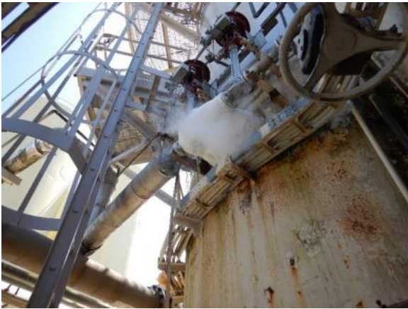
Photo 4-5. Ice forming on piping and tank wall is in VANDA Level 2 condition.
