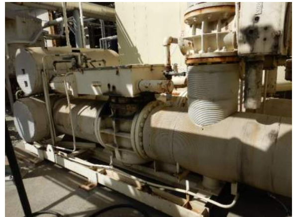
Photo 4-8. No significant corrosion was visible on the non-insulated areas of the switch valve .
