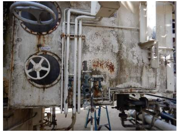
Photo 4-4. Side view of turbine duct box exhibits light corrosion. Underside is in VANDA Level 3 condition.
