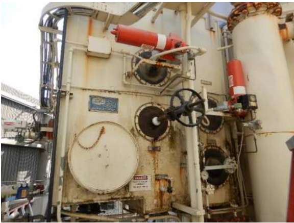
Photo 4-3. Light corrosion on the turbine duct on the northwest side of the cold box.
