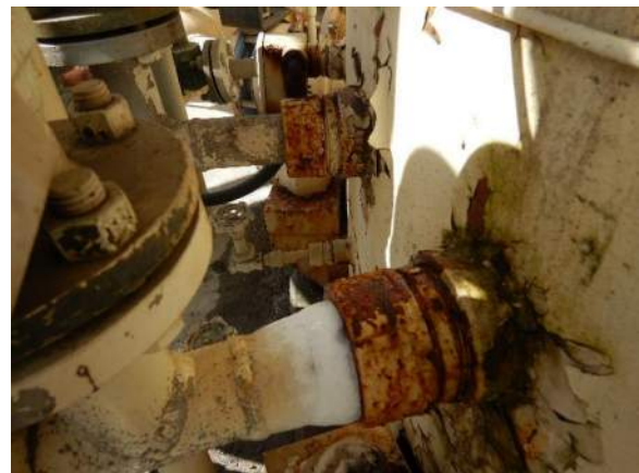
Photo 4-2. Typical coating delamination on the pipe penetrations and ice forming at the threads.
