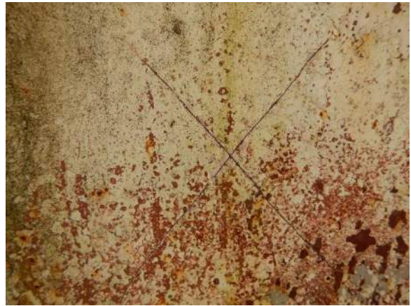
Photo 4-12. Coating adhesion test indicates a rating of 6 out of 10 per ASTM D6677.
