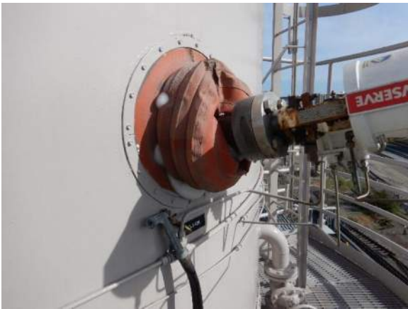
Photo 4-13. Ice forming on the valve at the second platform down from the top of the tank.
