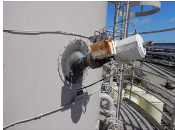
Photo 4-20. The tank shell is in good condition. Minor corrosion observed on the valve cover.
