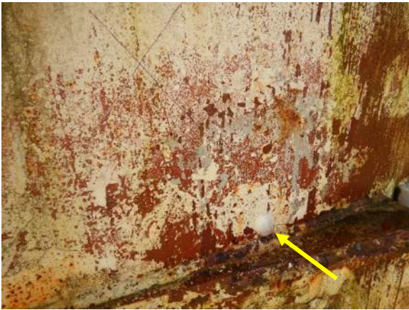
Photo 4-11. Ice forming on a pinhole leak and coating delamination surrounding it.
