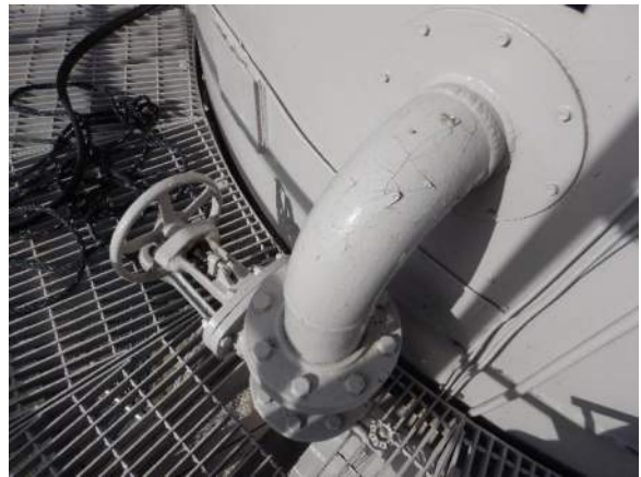
Photo 4-14. Cracked coating on an elbow at the second platform.
