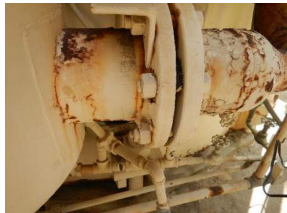
Photo 4-18. Detail view of the lower piping leading to the Thaw Heater.
