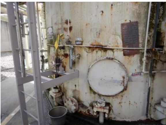
Photo 4-1. Lower north side of the tank shell exhibits coating delamination and light corrosion.
