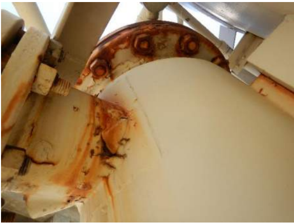
Photo 4-19. Coating failures on the surfaces of the upper pipe.
