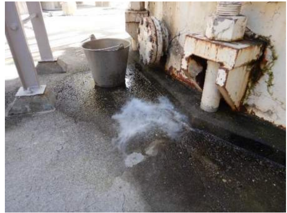
Photo 4-6. Melting ice has contributed to the light corrosion observed on the tank lower surfaces.
